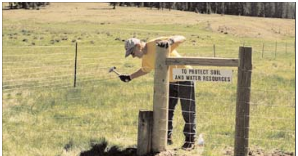
Volunteers installing cattle/ATV riparian enclosure to protect the riparian and water resources of the headwaters of Bitter Creek
