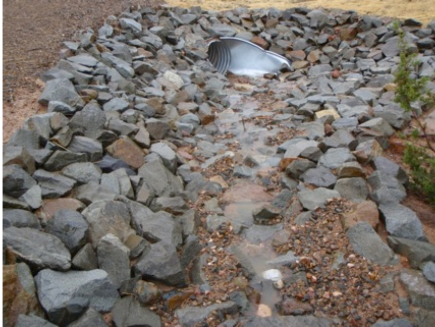
Rock Splash pad under culvert disperses force
