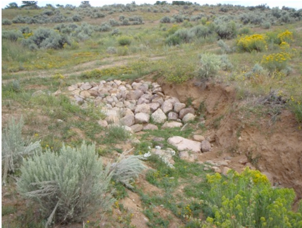
Gully formed by road, rock structure protecting road from headcut
