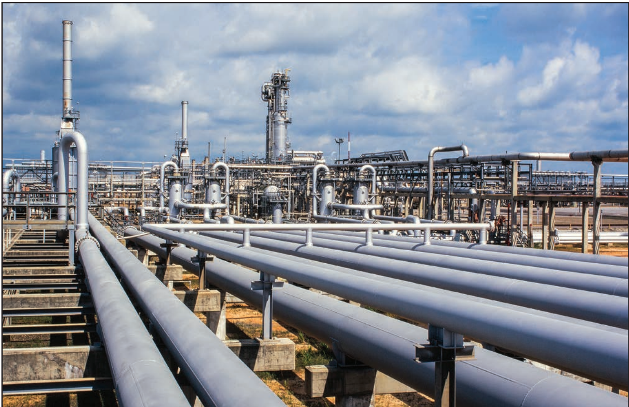
Williams Field Services Processing Facility, Bloomfield, NM. Photo courtesy of Ecoflight, and ecoflight.org. 463
