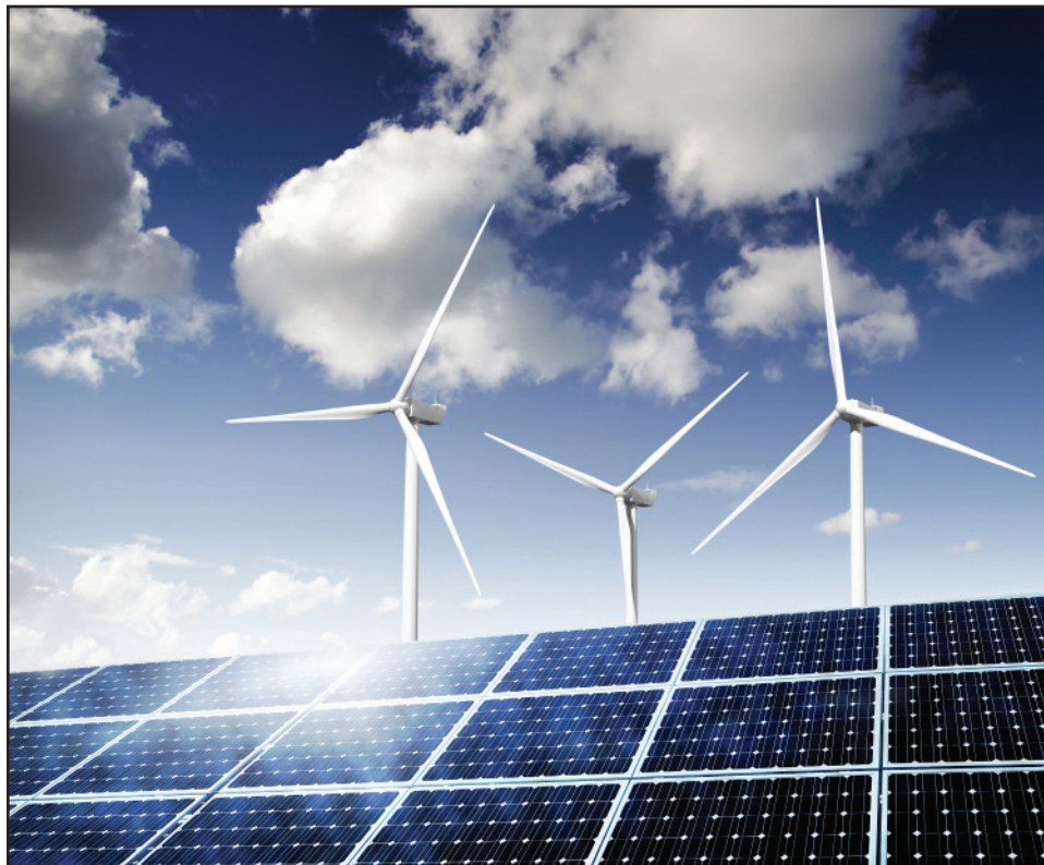
Solar Photovoltaic (“PV”) Array at Wastewater Treatment Plant in Northern New Mexico 596
